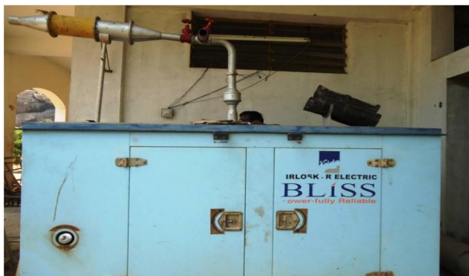
Figure 8. Diesel Genset Mounted with \text{CO}_2 Absorption Chamber
