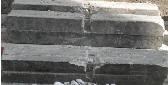
Figure.2. Honeycomb edges are chipped off
