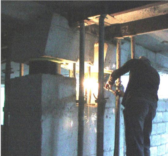
Figure 18. The moment of cutting of the vertical reinforcing bars of existing column
