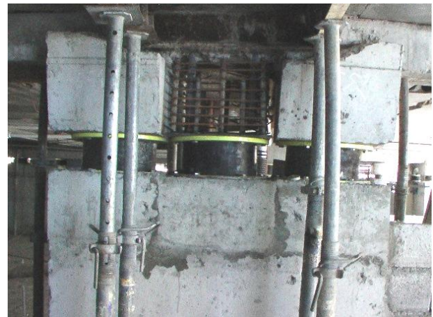
Figure 20. Concrete is casted under the lower socket of the middle seismic isolator and the upper socket and hooks are installed above it which are fixed with the spacing of 50 mm
