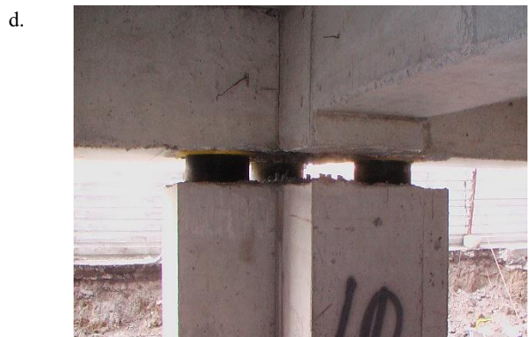
Figure 26. Views of the reinforcement cages of the newly designed upper pedestals and upper beams (a, b); after concrete of upper pedestals and beams above the isolation interface is casted the process of cutting of the reinforcement bars of existing columns is going on (c); final view of the joint where the existing column is cut, and the superstructure is isolated (d)
