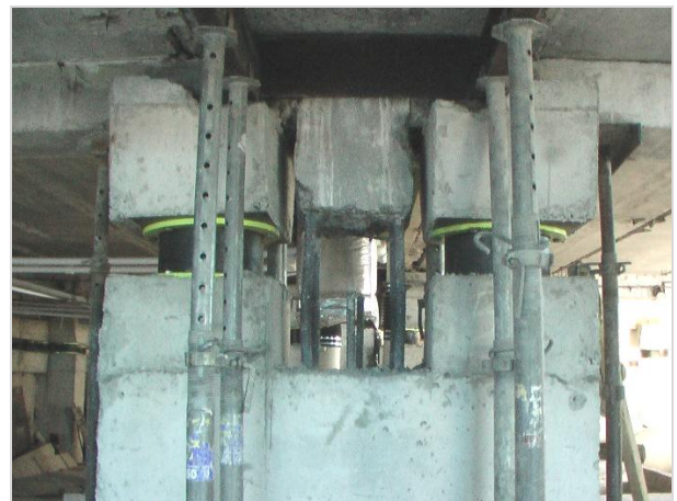
Figure 17. Buckling of the existing column's vertical reinforcing bars after removing of a part of the column's concrete
