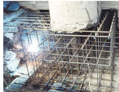
Figure 12. Temporary support under the one half of the existing column section (a), and the temporarily supported existing column and the wall behind it with the reinforcement frame of the upper pedestal installed (b)
