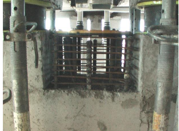
Figure 19. Installation of the hooks and the lower socket under the middle seismic isolator after cutting of the vertical reinforcing bars of existing column
