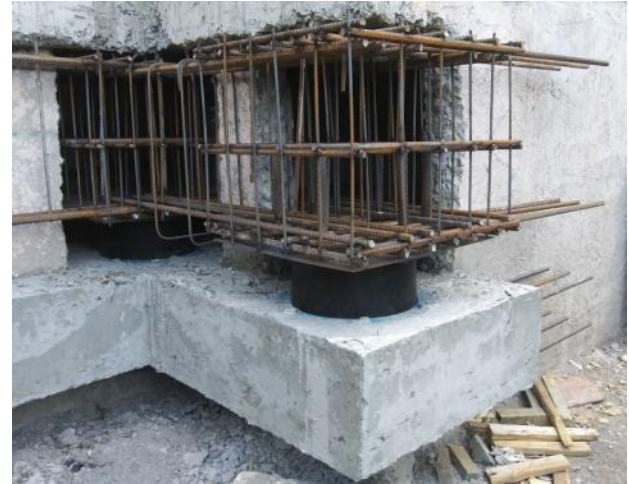
Figure 36. One of the stages of installation of seismic isolation in the basement of existing 9-story large-panel building in accordance with the Patent of the Republic of Armenia № 579
