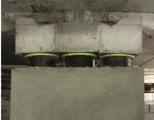
Figure 21. Concrete is casted above the upper socket of the middle seismic isolator and all the temporary supports are removed
