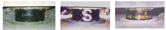
Figure 4. General view of the existing 5-story stone apartment building retrofitted by base isolation (a) and fragments of its isolation system (b)
