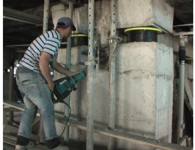
Figure 16. Concrete is casted on the parts above the upper sockets of isolators to support the superstructure and the process of cutting of the existing column starts after the concrete above the isolators gets its design strength
