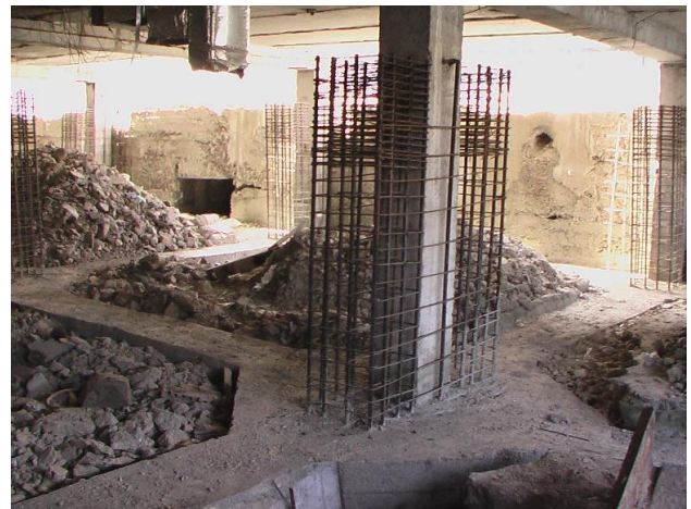
Figure 14. Newly designed mutually perpendicular strap beams connect the existing spread footings of the basement columns and the reinforcement cages of newly designed columns are anchored in them
