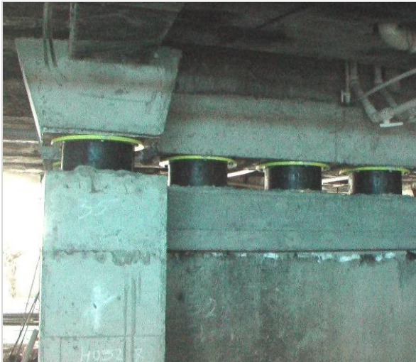
Figure 22. Fragment of the already cut shear wall and the adjacent column with the installed seismic isolators
